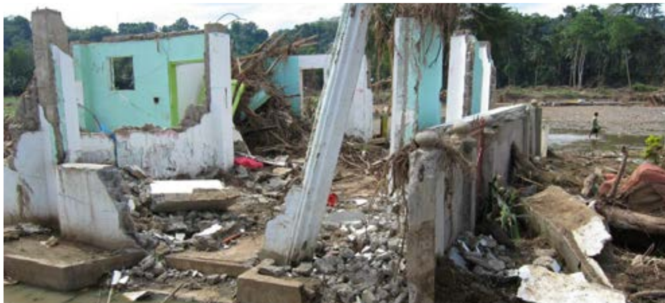
Destruction left after flash floods following Tropical Storm Washi Photo by Charisse Mae Borja
