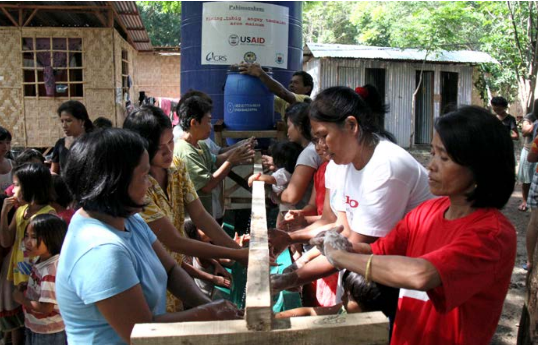
Clean water supply and taps installed at transitional settlement sites Photo by Jennifer Hardy/CRS
